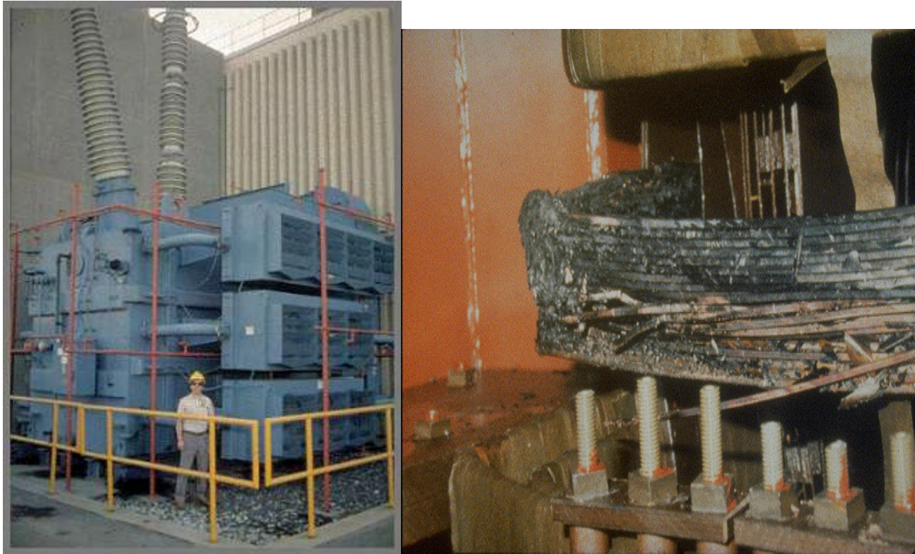
Figure 3. Generator step-up transformer owned by the Public Service Electric and Gas Company of New Jersey damaged by 13-14 March 1989 geomagnetic storm. Images provided courtesy of Public Service Electric and Gas and Peter Balma.
